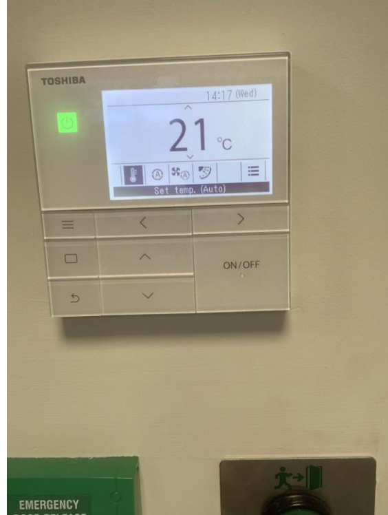
Zone control panel
