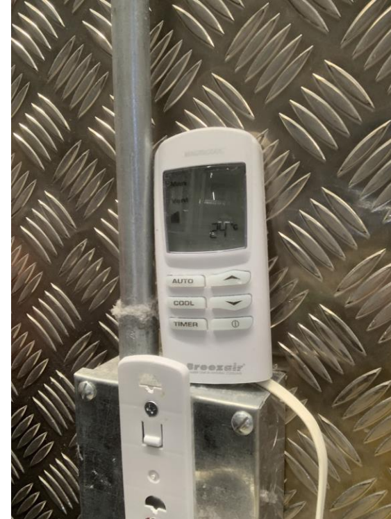
Production cooling control
